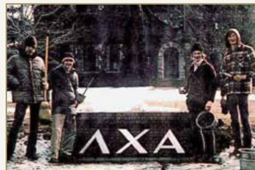
Dale Miller '73 X985, John Crook '72 X980, John Stirniman '76 X1033, and Brian Parkinson '76 X1035 building the AXA sign at the front of the chapter house. John Stirniman was the designer and coordinator for construction of the sign as an associate member class gift for the class of 1979.
